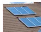
Solar thermal hot water
