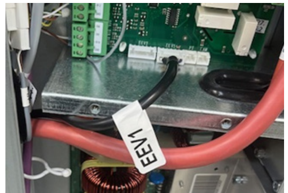
Fig. 67: Expansion valve cable
